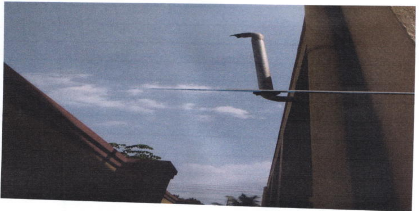
DG set chimney
